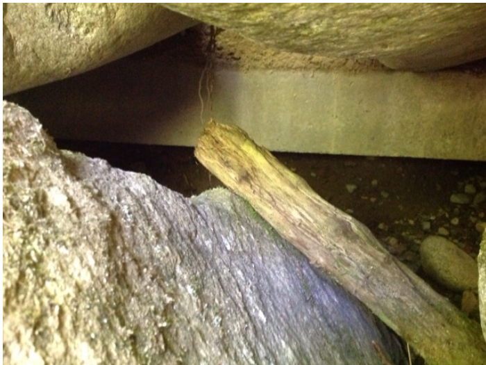
scoured footings right approach - approx 500mm from front face
