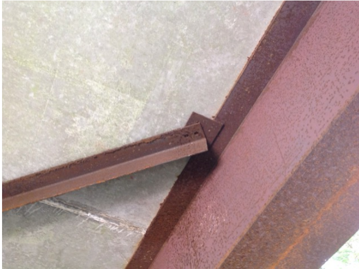
missing bracing bolts
